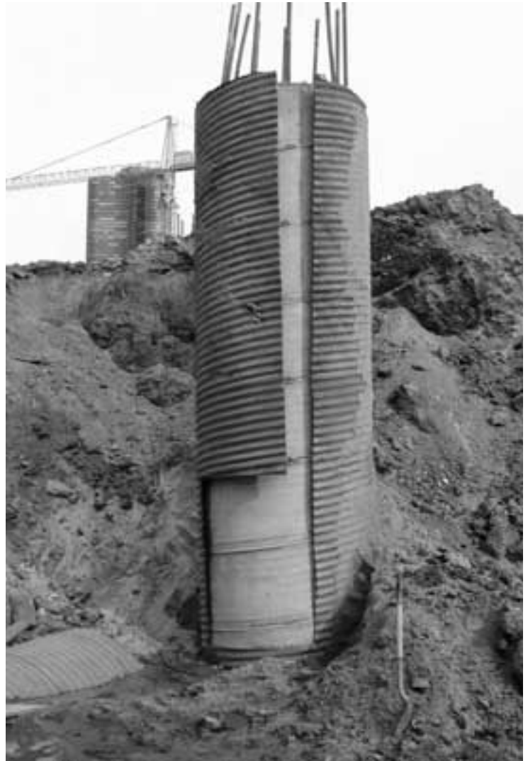
Drilled Shafts become below-grade columns once the double-walled CMP liners are removed.
