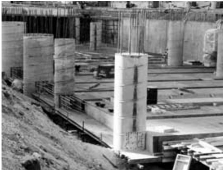
Lower level 1 framing and floor slab construction. Note drilled-in connections at caisson/beam intersections. Slurry wall in background designed to cantilever until Level 1 construction is complete.
