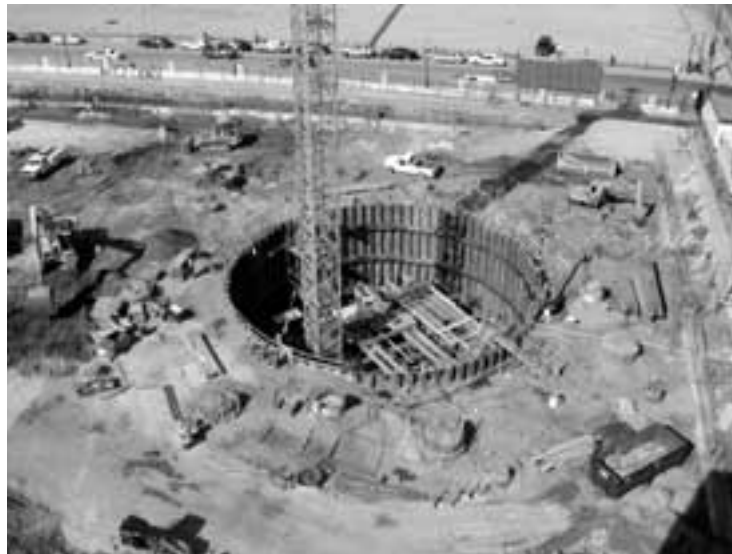
Sheet pile cofferdam braced by compression rings enabled tower core and shear walls to be constructed early.
