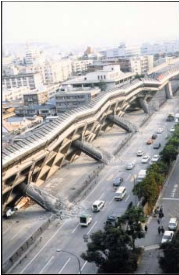
Photograph-1.1 Hyogo-ken Nanbu Earthquake
