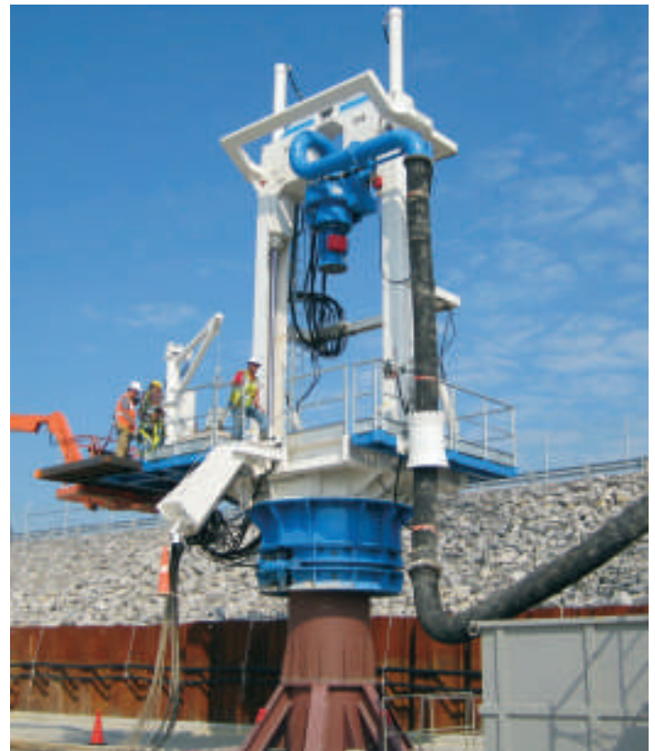
The Wirth drill being installed atop casing bolted to the work platform at surveyed locations
