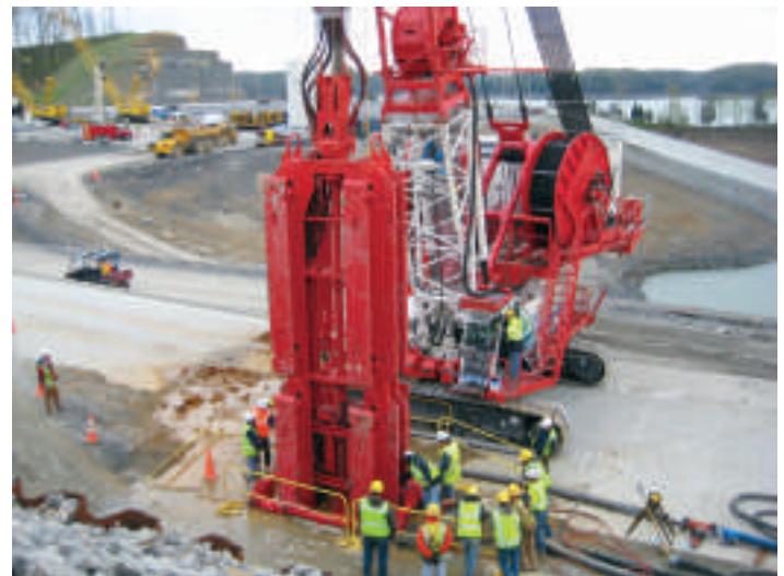
The hydromill is inserted into a steel guide frame locked into guide walls on the work platform, allowing the mill to begin excavation at the right location in a vertical position
