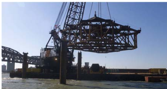
Benicia-Martinez Bridge Template being Hoisted Into Place As Shown By Speaker Richard Foley, P.E. of CalTrans.
